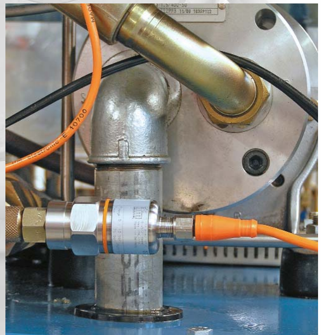
Pressure monitoring in hydraulic systems.
