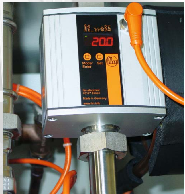
Ultrasonic flow rate measurement in a water circuit for quantity monitoring.
