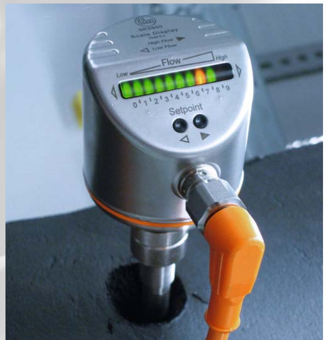
Flow monitoring in a return pipe with a large nominal width.
